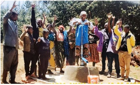
Well # 0766 was installed on 10/6/2022 in the village of Makogo, Tanzania and will serve 60 people.
